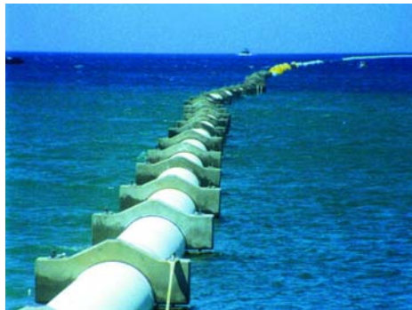
Figure 10 Sea water in-take pipes ( www.reinforcedplastics.com )
