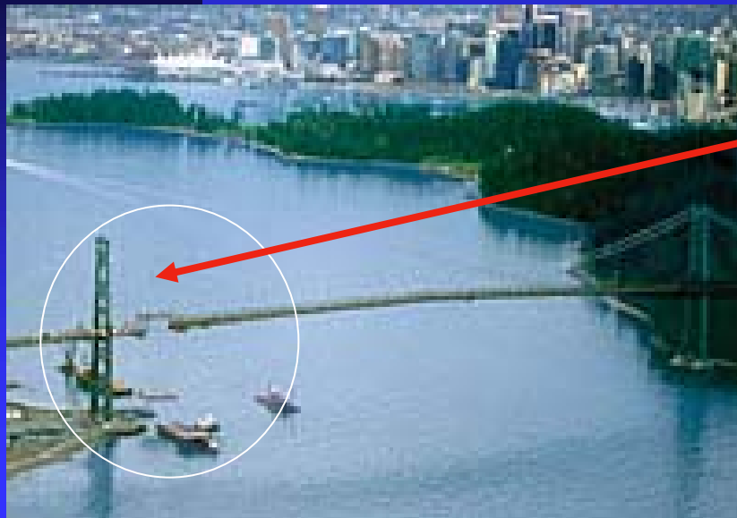
The Lions Gate Bridge (Vancouver, British Columbia, Canada) truss and deck sections were replaced during 10-hour night closures.
